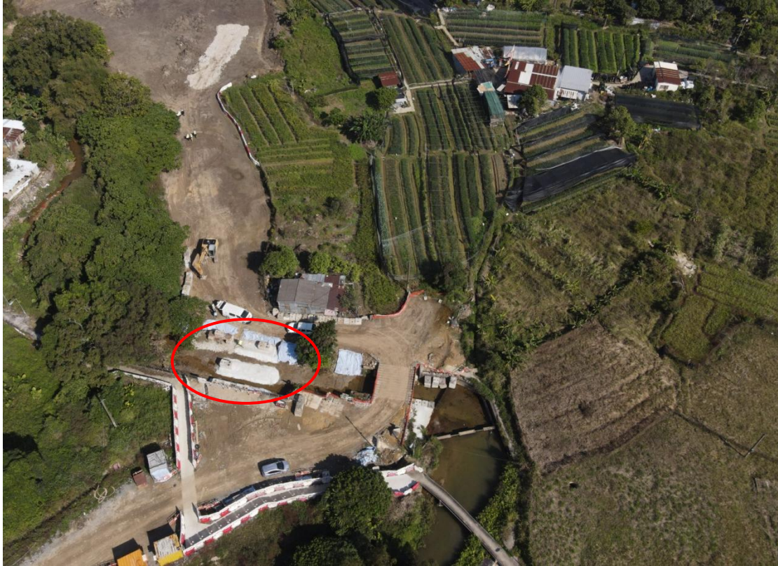
Figure 2 During construction of a temporary bridge for the main road in Agri-Park Phase 1, some concrete foundation (circled in red) was once formed at the stream bed
